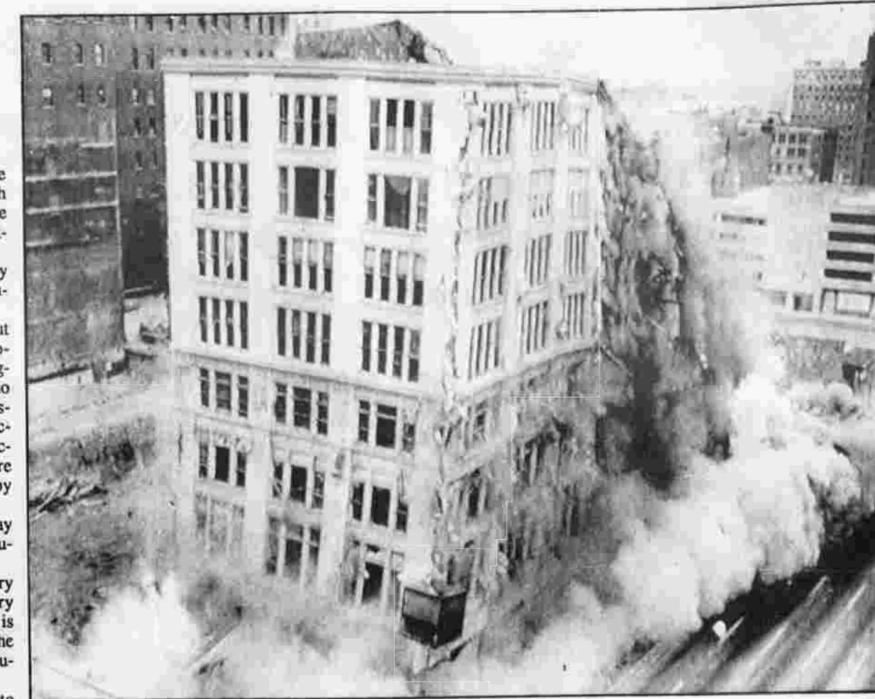
COMING DOWN — The 75-year-old Occidental Building crumbles as it is intentionally imploded Sunday to make room for a new mall in downtown Indianapolis. The building was brought down in seven seconds by 361 charges of explosives.
